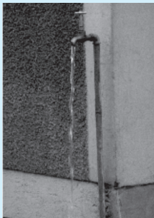
Picture 9.1. Water dropping from pipe
