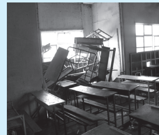
Picture 5.2. Improperly handled school properties
