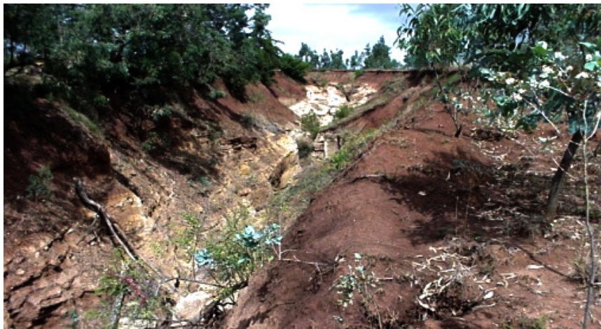
Figure 6.16: Severe rill and gully erosion due to improper land use.
