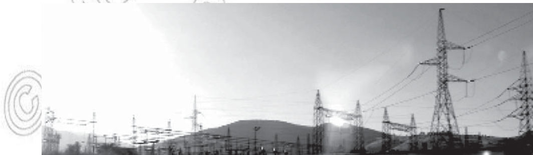
High voltage power lines and pylons
