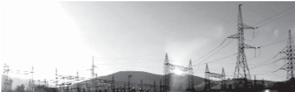
High voltage power lines and pylons
